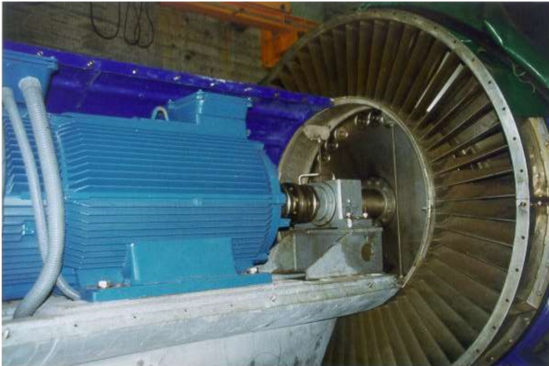
Turbine and generator in Wave Power Plant Cachorro, Pico, Azores 1998
