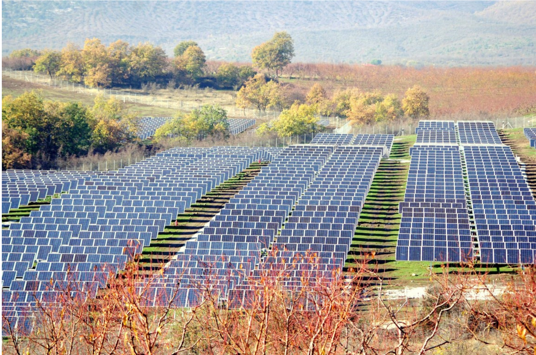
8 MW PV plant using horizontal single axis tracker, Greece
